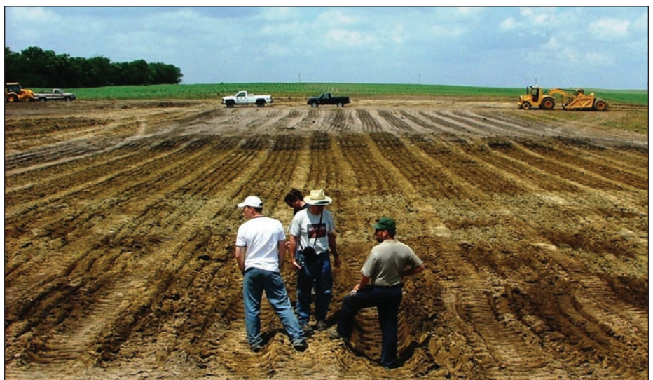
Wetland construction on a family farm near Lexington, Illinois. Photo courtesy of Tim Lindenbaum, The Nature Conservancy.
